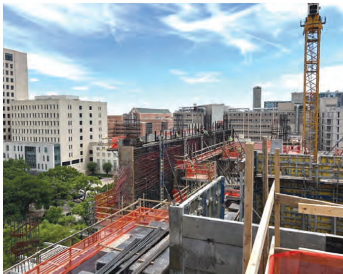
Fig. 6. Careful coordination and placement of rebar and tendons helped mitigate congestion. (Photo courtesy of Vaughn Construction.)
