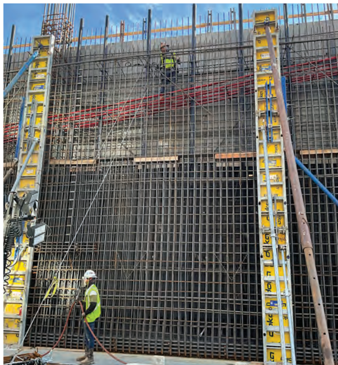
Fig. 5. Walter P Moore worked closely with Suncoast Post-Tension to determine the exact tendon layout.
