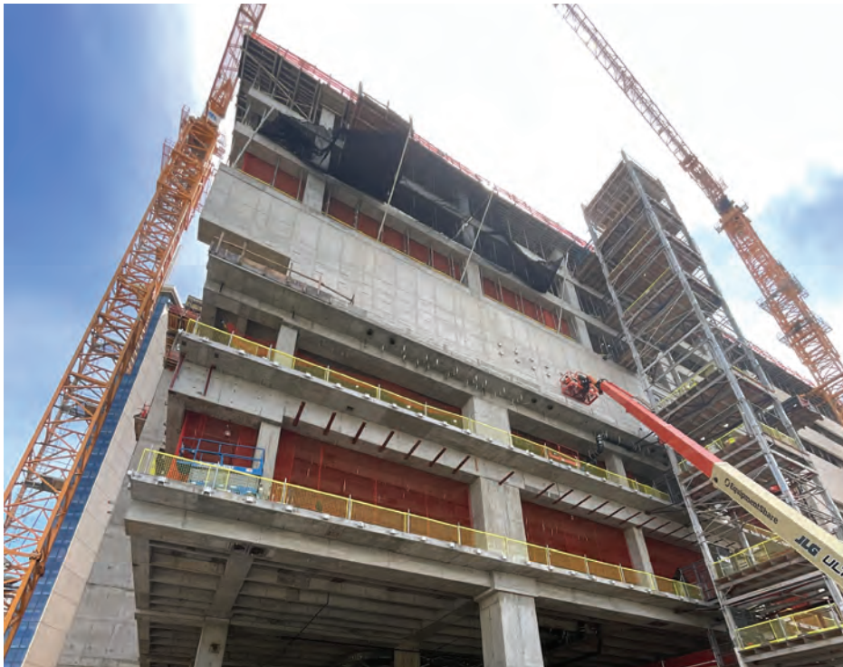
Fig. 8. The temporary supports were removed once the upper level transfer girder was ready to support the load.
