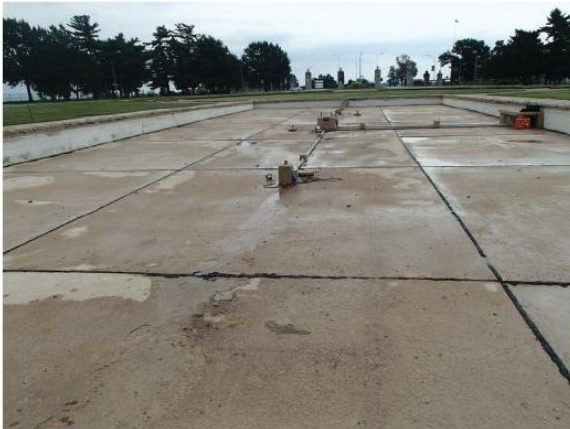
Fig. 2: Concrete spalling at fountain slab
