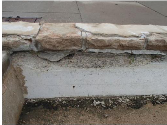
Fig. 4: Concrete deterioration at original concrete walls
