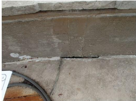
Fig. 8: Gap between basin floor and perimeter wall
