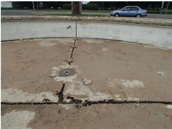
Fig. 3: Close-up of concrete spalling at fountain slab
