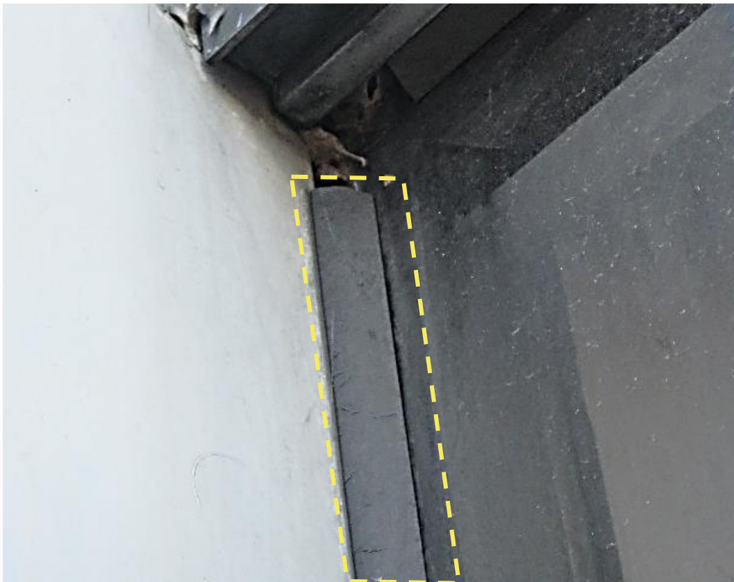
Figure 3: Example of gasket cracking deterioration at a 1965 curtain wall system
